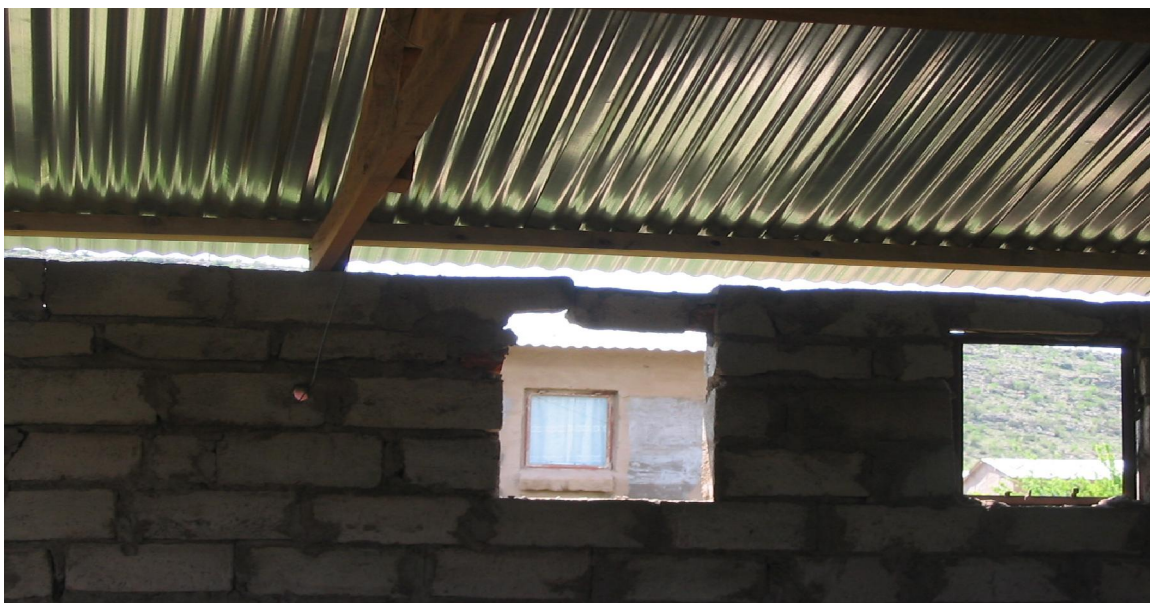
FIGURE 17 : CONSEQUENCES OF NOT USING A LINTEL OR REINFORCED U-BLOCKS
